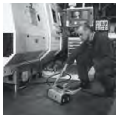
Lifting a machine with a cylinder and air hydraulic pump with remote control.
