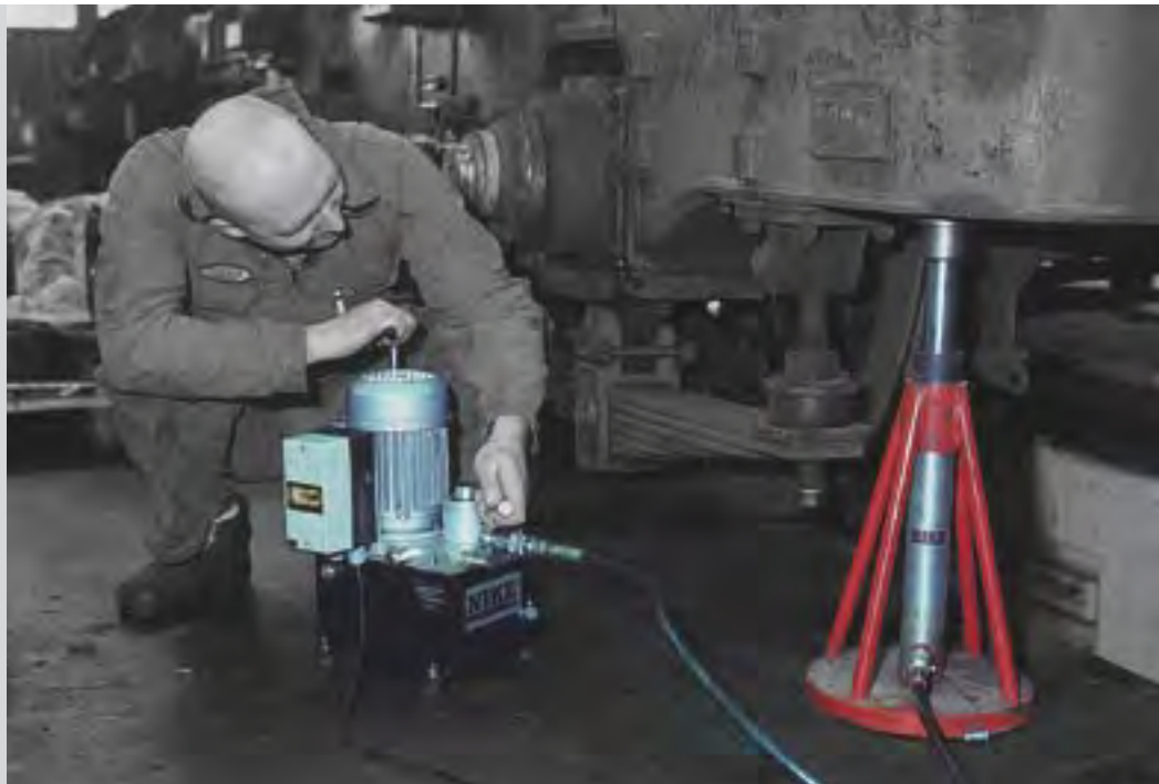
An electric pump and cylinder being used to lift a locomotive for maintenance.
